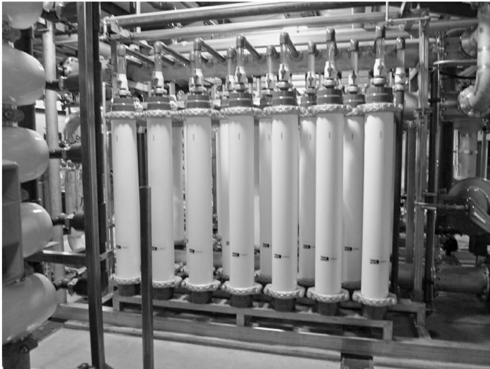
FIGURE 8.21 Ultrafiltration skid showing clear permeate piping.
